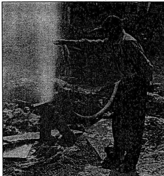
A member; of the medical center, maintenance staff inspects the yield of a new bore hole before it is capped and connected to piping. .'
